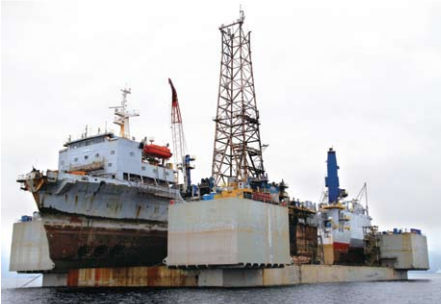
The jumboisation of Noble Leo Segerius was carried out at sea with the front of the ship first secured to the floating dock, FS-1, and submerged to receive the stern block afloat
